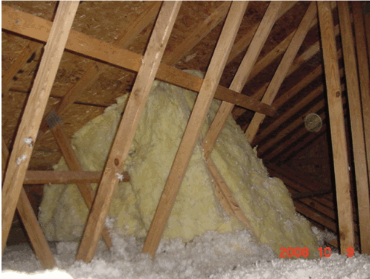
Photo 7 - The fiberglass insulation on the skylight shaft will need removal to seal the gypsum board seams using spray foam insulation. Then re-apply R-19 (6" thick fiberglass batt), 2 layers (minimum).
