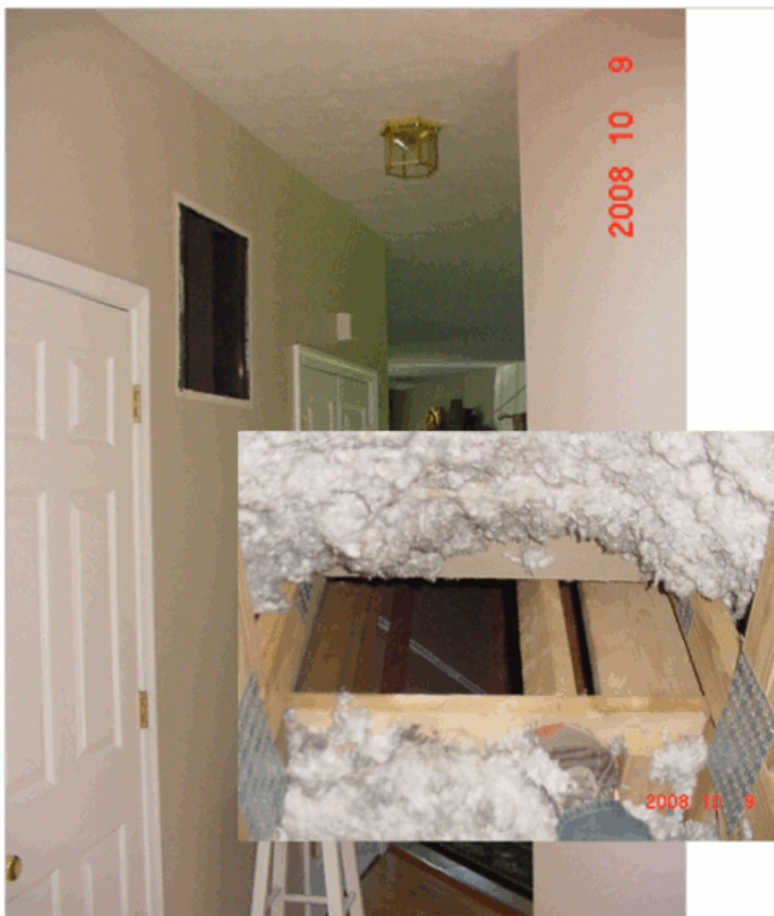
Photo 8 - With the return air grille removed, it was revealed that the attic space is totally open to the conditioned space, as can be seen in the inset photo taken from the attic looking down on the ceiling. This opening must be sealed using a plywood or gypsum cover cut to fit and sealed.
