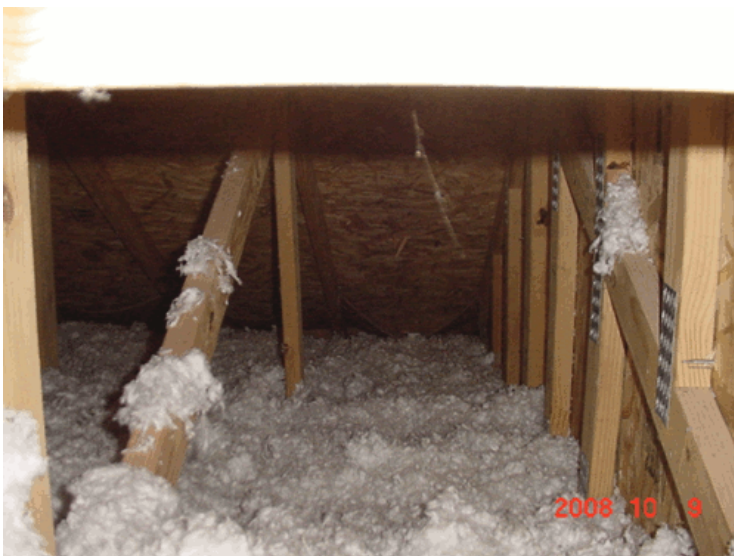
Photo 6 - Existing blown insulation is an average 10 inches thick. However, the effective R-value is estimated to about nine inches. Adding more insulation to achieve R-38 or better will exceed today's code requirements. R-50 is not unreasonable and is in line with Energy Star recommendations. It is also recommended to add rafter vents
