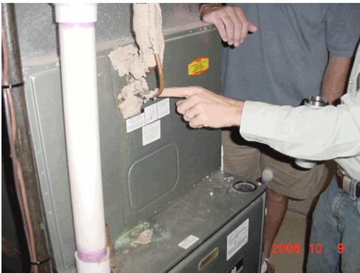
Photo 5 - The insulation used on the suction line for the AC is haphazardly installed. This should be removed and replaced with a foam insulation to match the existing black foam. Include a short piece on the liquid line at the housing.
